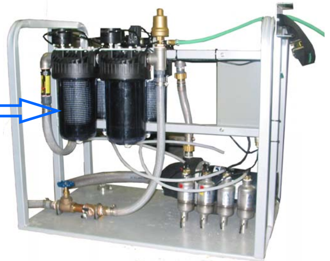
The Gas Transfer Module within the gPRO system, this particular system is a gPRO HP4 (there are 4 modules, 2 are not shown)
